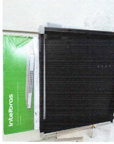
RACK E SWITCH
